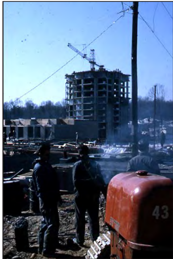
Figure 17. Heron House high-rise apartment building under construction in 1964 (George Mason University Libraries [GMUL] item ID C0001B113_01).
