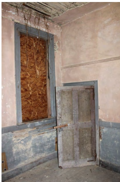
Figure 6, detail of hinge configuration with the “H” arm of the hinge concealed behind the architrave, first floor, northwest room, Elizabeth Lipford, DHR archives photograph, 2021
