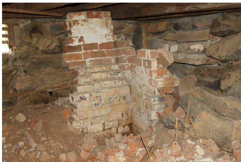
Figure 5, cellar, portion of brick veneer wall with pargeting and paint, Elizabeth Lipford, DHR archives photograph, 2021
