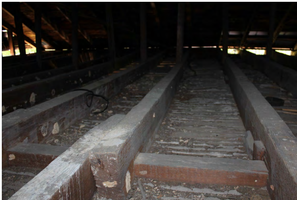
Figure 9, attic floor framing. Note principle girder on the right side of the image and overlapping joists on the left side of the image, Elizabeth Lipford, DHR archives photograph, 2021
