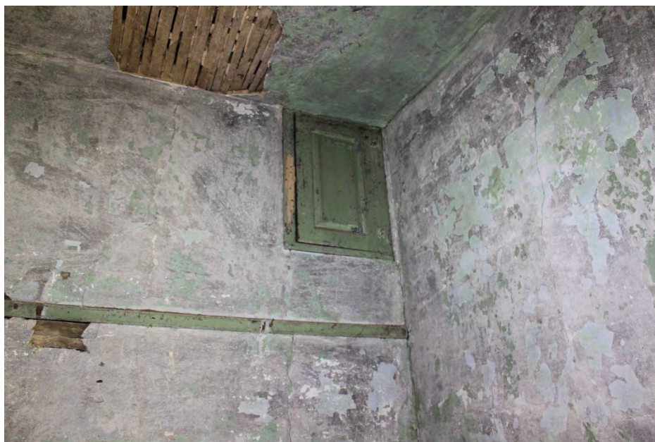
Figure 8, storage cubby under stair landing, accessed from northeast chamber, first floor, Elizabeth Lipford, DHR archives photograph, 2021
