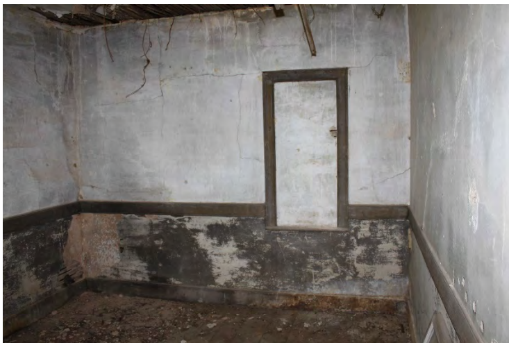
Figure 4, Northeast chamber, second floor, original window opening enclosed when the wing was added on the east elevation, Elizabeth Lipford, DHR archives photograph, 2021.
