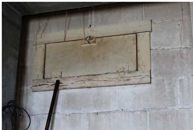
Wooden doors for cables, rear wall, 1947 transmitter building. Photo by Elizabeth Lipford, 2021, DHR Archives
