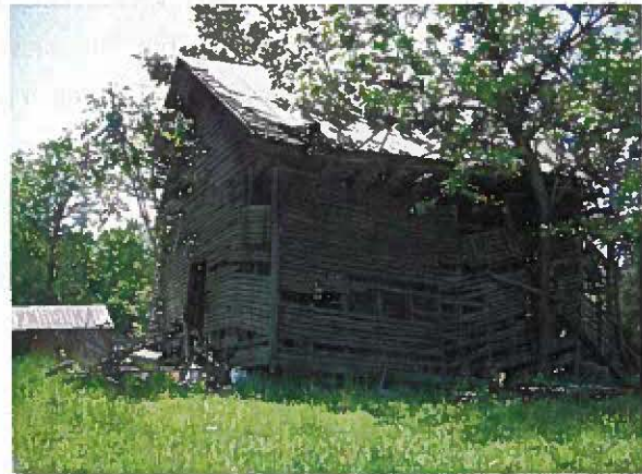
Photograph 10. The deteriorating Granary
