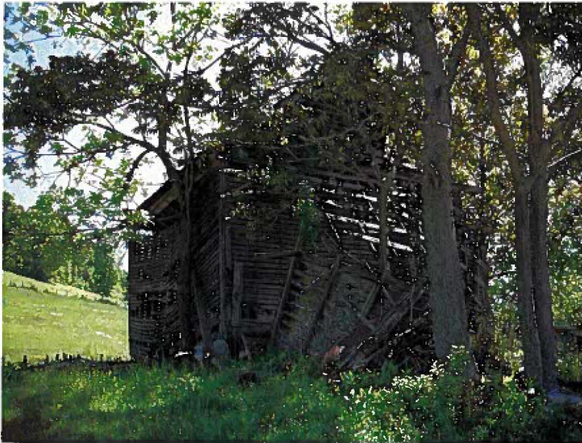
Photograph 11. A Shed addition to the Granary has collapsed
