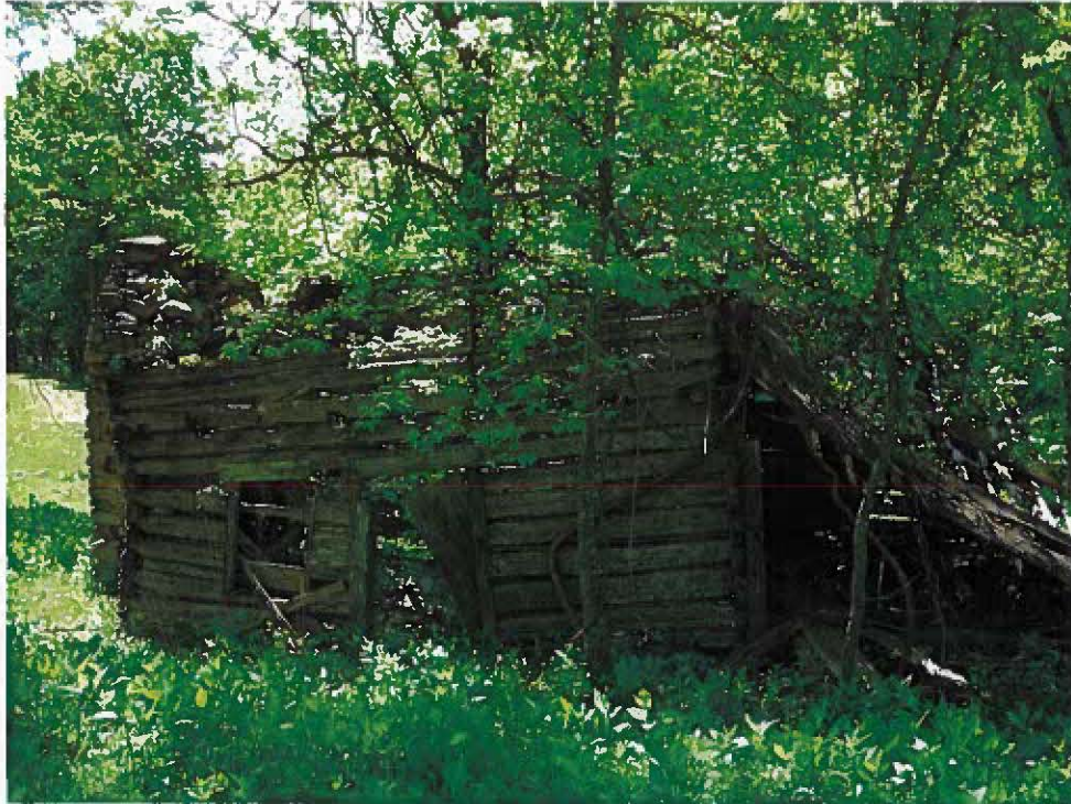
Photograph 14. The Slave Cabin and its Collapsed shed addition
