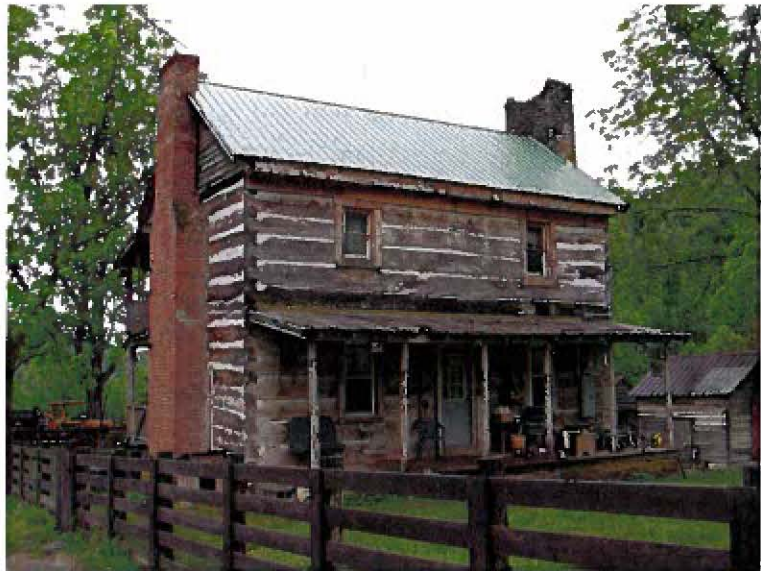
Photograph 2. The Façade prior to window installation in the gable end and repairs to the front porch, where ghost lines of the former entry are evident
