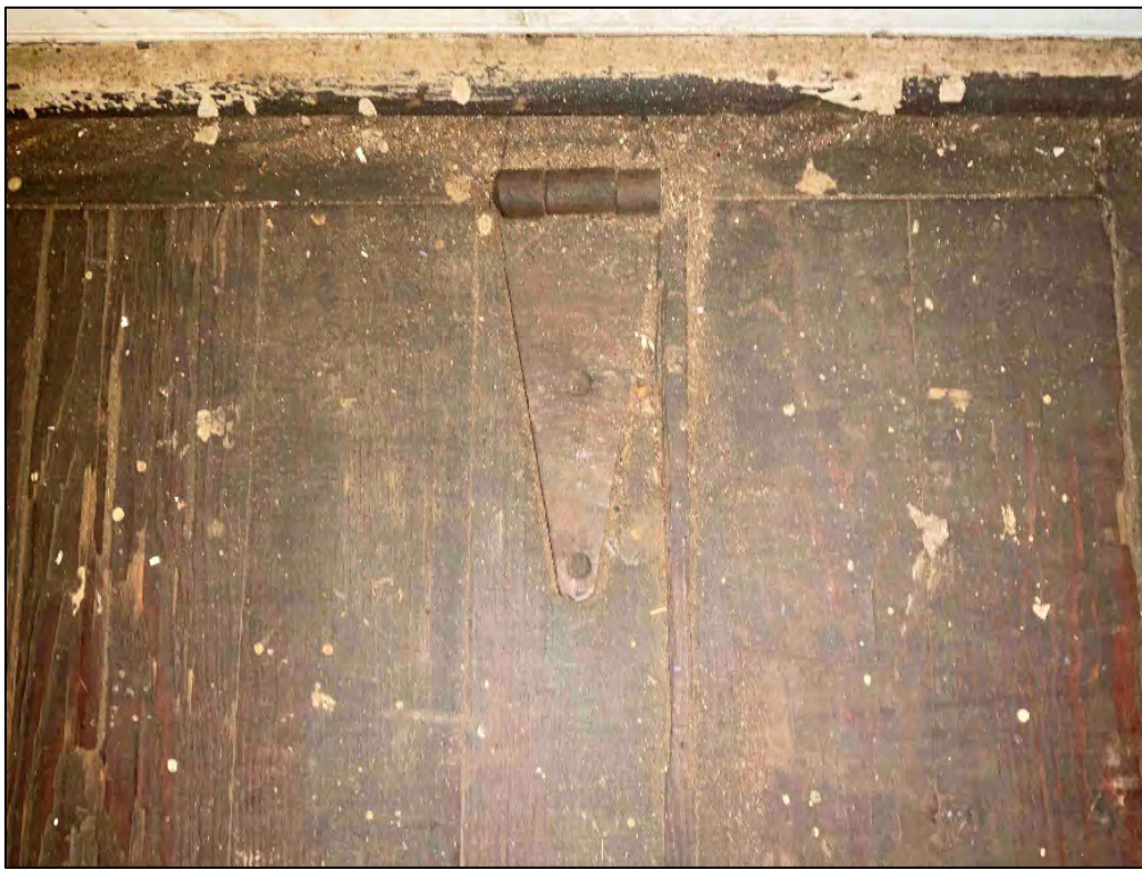
Building A, interior, north classroom, hinge on stair hatch. March 2022. Photo by J. Lahendro.
