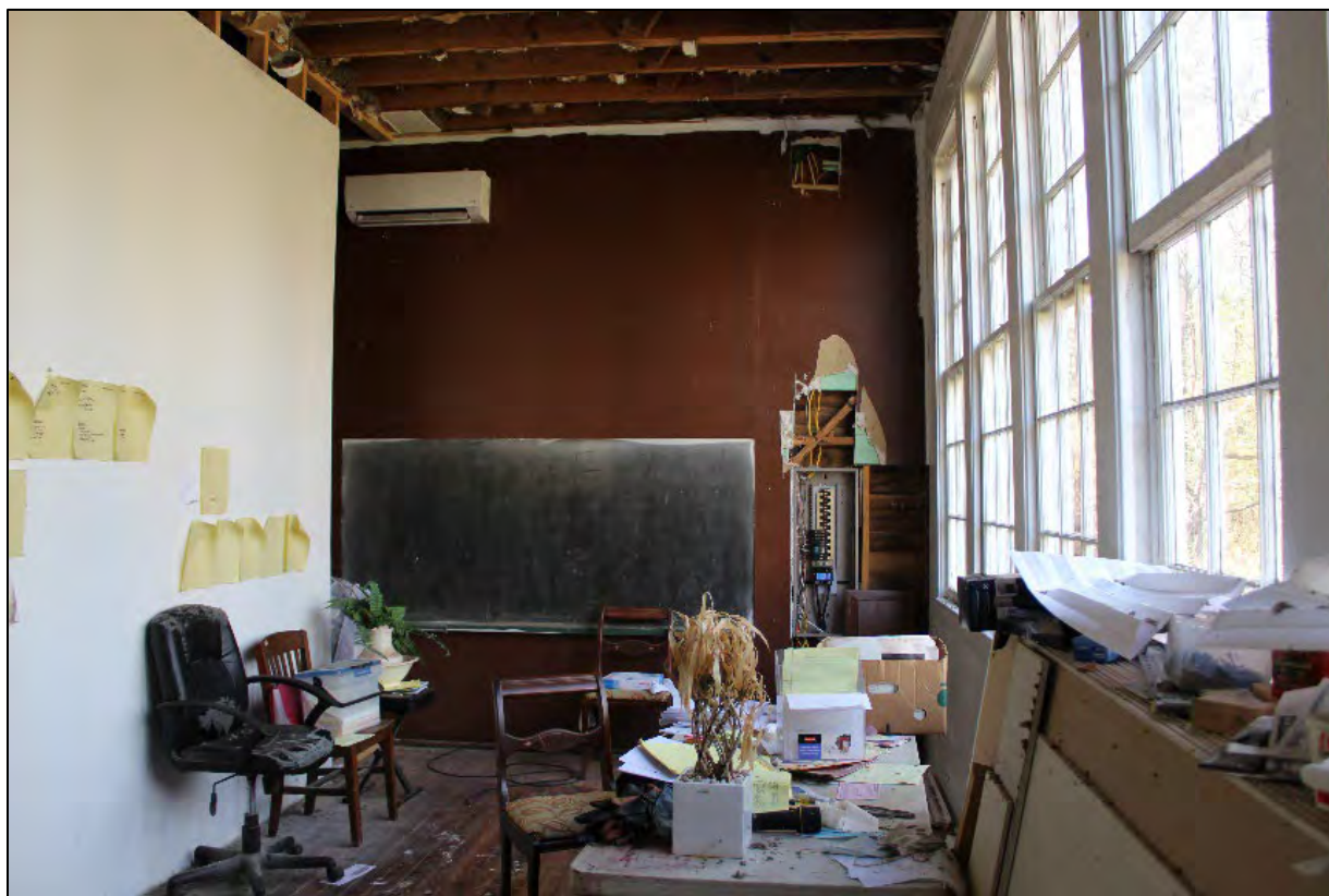
Building B, interior, south classroom, original windows and blackboard. Partition wall on left in photo is nonhistoric. December 2021.
