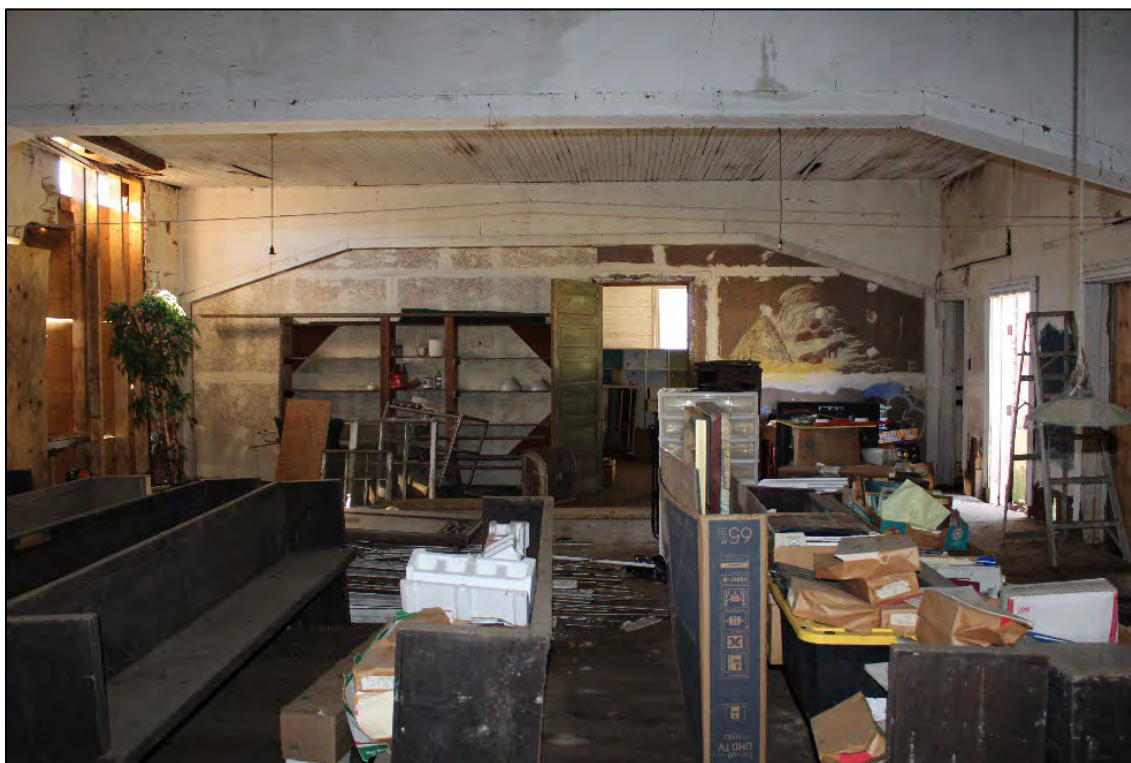
Building A, interior, looking from north classroom through center classroom. Cased openings are visible, as is a new wall constructed between the southern and central classrooms. The door in the new wall is believed to be an original sliding door from the school that has been reused. December 2021.
