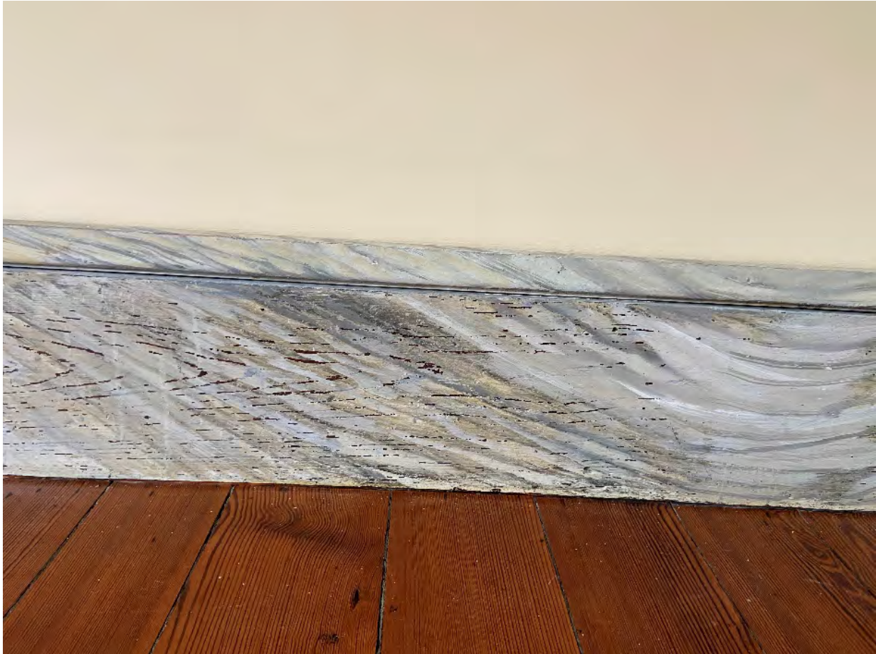
Figure 6 A section of the east room's baseboard retains the original nineteenth century marbling.
