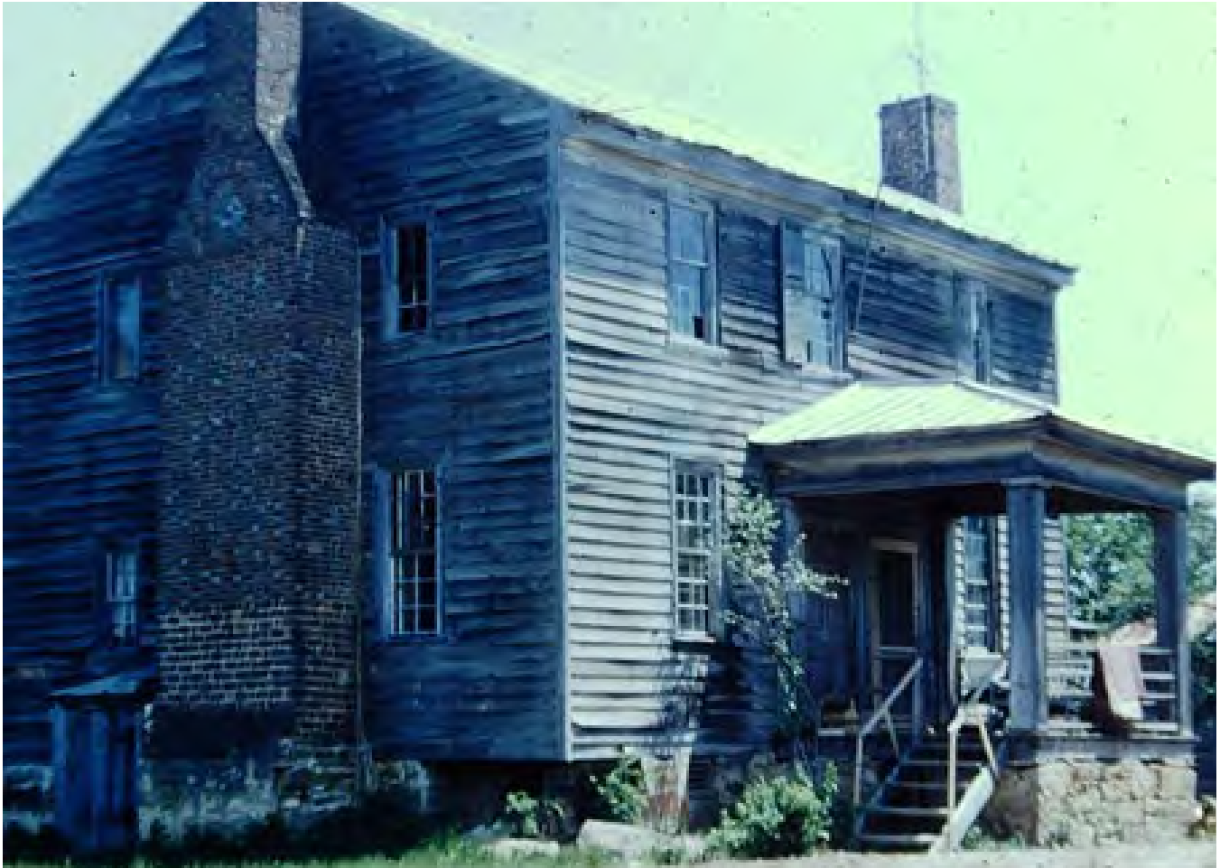
Southwest corner from southwest showing missing section of foundation, 1960s. A earlier basement entry is visible beside the chimney [Collection Old Brunswick Circuit Foundation].
