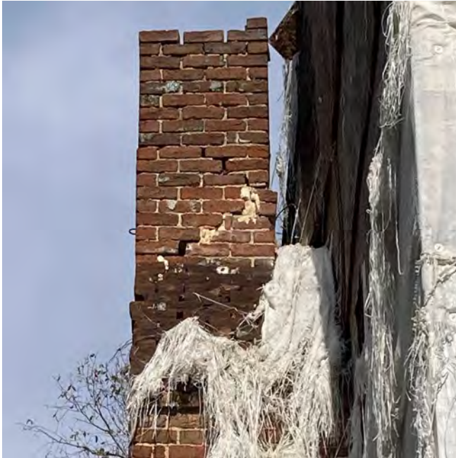
West chimney shaft looking north (left) and east chimney shaft looking north (right).
