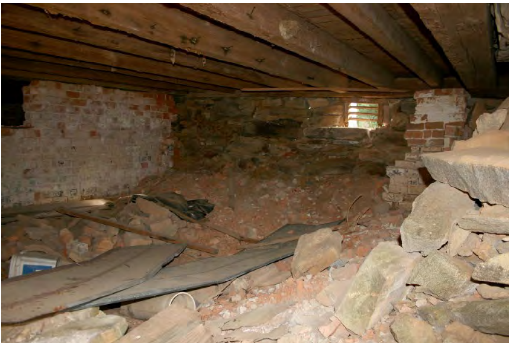
Basement, West Room, looking southeast showing central brick cross partition (left). Added brick bulkhead on the right.
