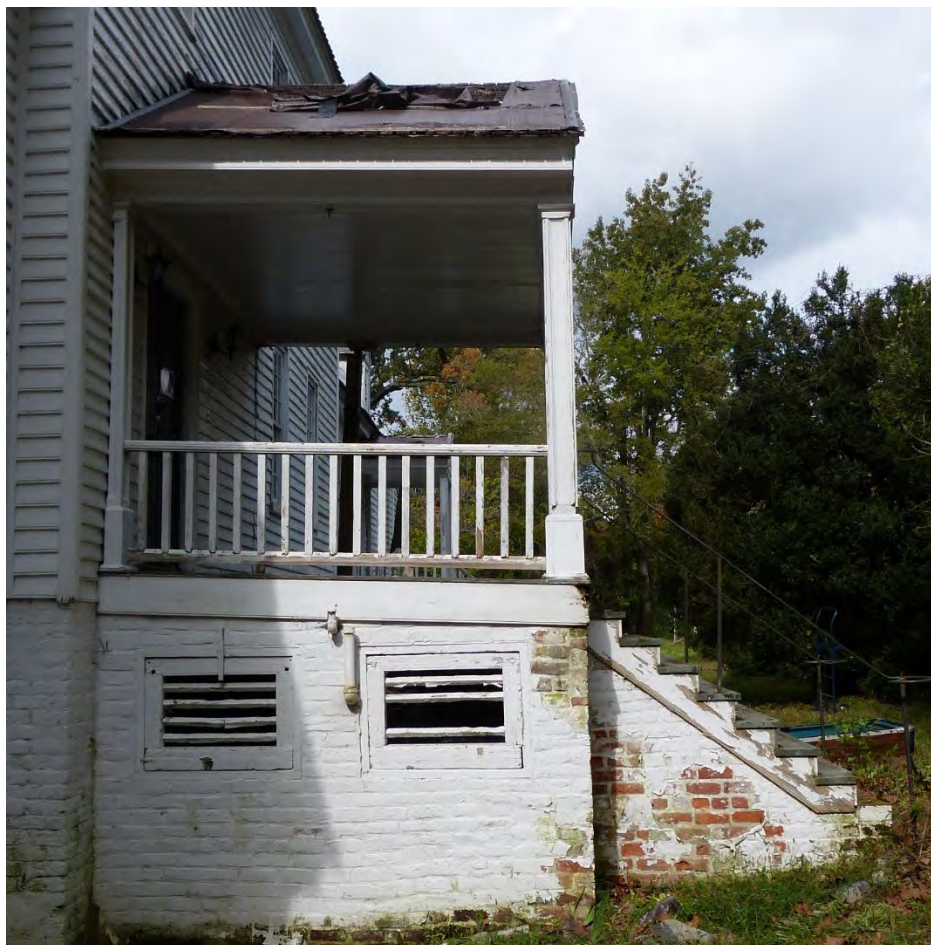
Figure 5: Wood slat windows in the mid-twentieth century porch base may have historically been cellar windows on the west elevation of the Period I basement.
