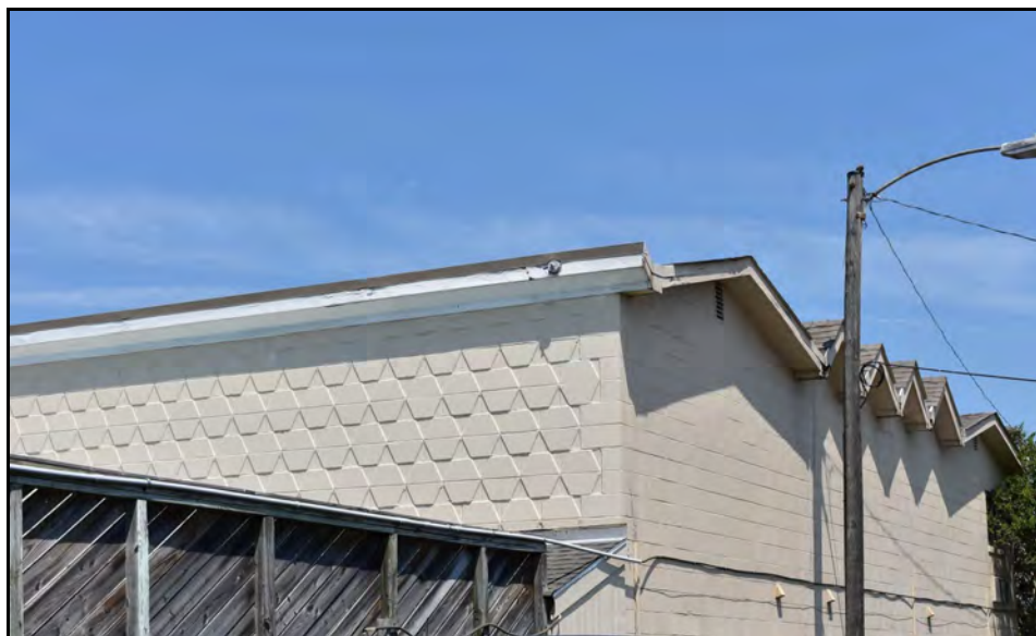
Figure 2. Looking northwest at the east (right) and south (left) elevations of the original guest room wing. Note folded-plate roofs extending to the east and the honeycomb concrete tile cladding on the south elevation. The later frame fence around the pool area is seen in the lower left.
