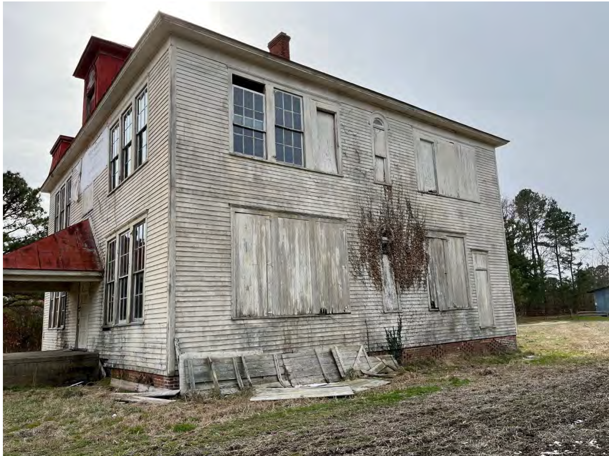
Installing refurbished windows on second story north side Photographer Marian Veney Ashton
